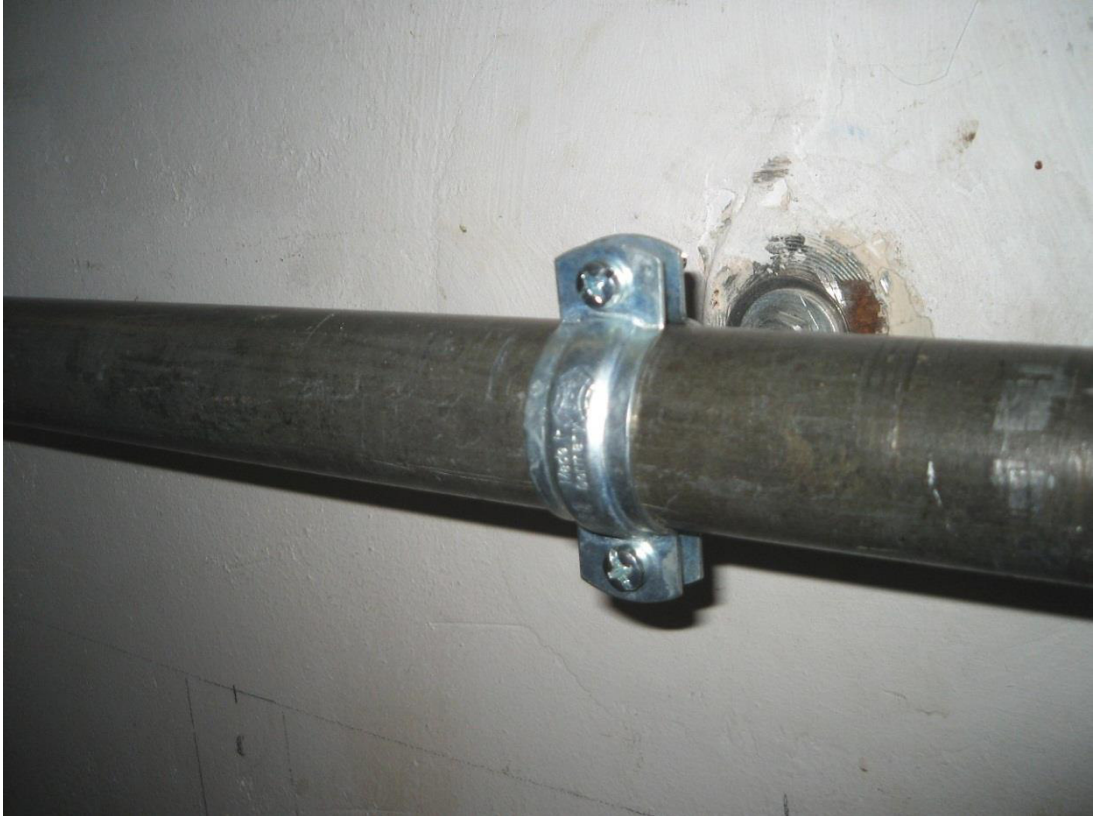
Fig. 1: Reference measurement: rigid fastening, measuring pipe diameter 33,7 mm, 1"
